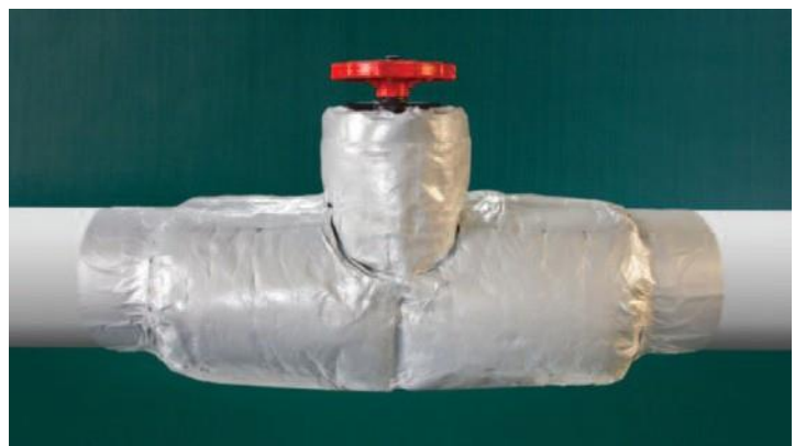
Figure 13 — Finished insulation. All seams are tightly sealed with tape and penetrations are tightly sealed with silicone caulk
